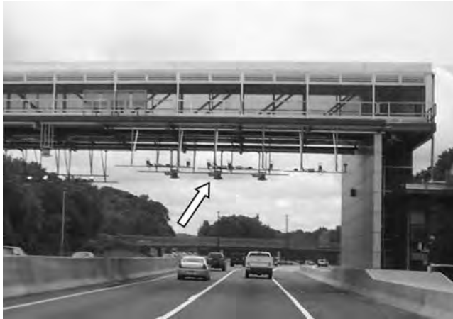
Figure 24.10: E-ZPass high-speed toll plaza—antenna array
